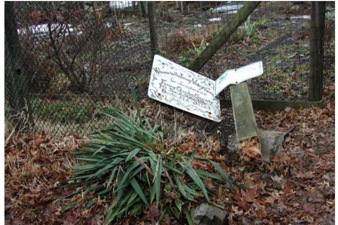
The corner fence post, and Fenway Garden Society sign shown rotted and snapped at the base.
